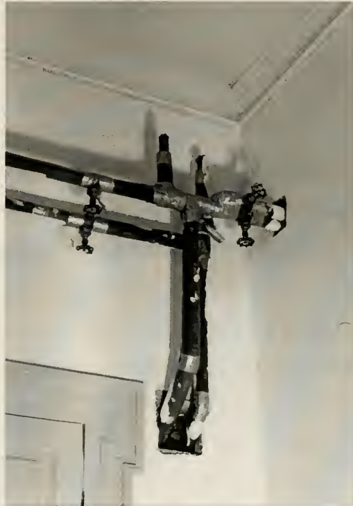
Figure 31 Destruction of Building Fabric Due to Inappropriate Mechanical System, 1998 Photograph by Author
